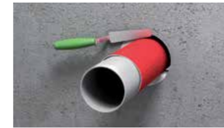
2. Ensure smoke tight seal of the annular hole (e.g. with Pacifyre® FPM Fire Protection Mortar or Pacifyre A Fire Protection Acrylic Sealant)
